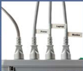
Cords and Cables
