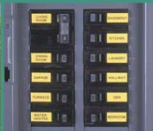
Safety Identification - Fuse box
