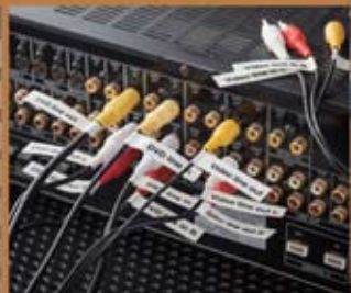
Wires and Cables
